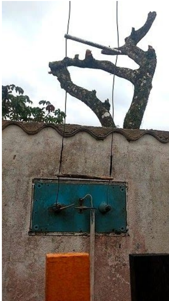
Photo: Detail of the output of the transmission lines of the coupler box
