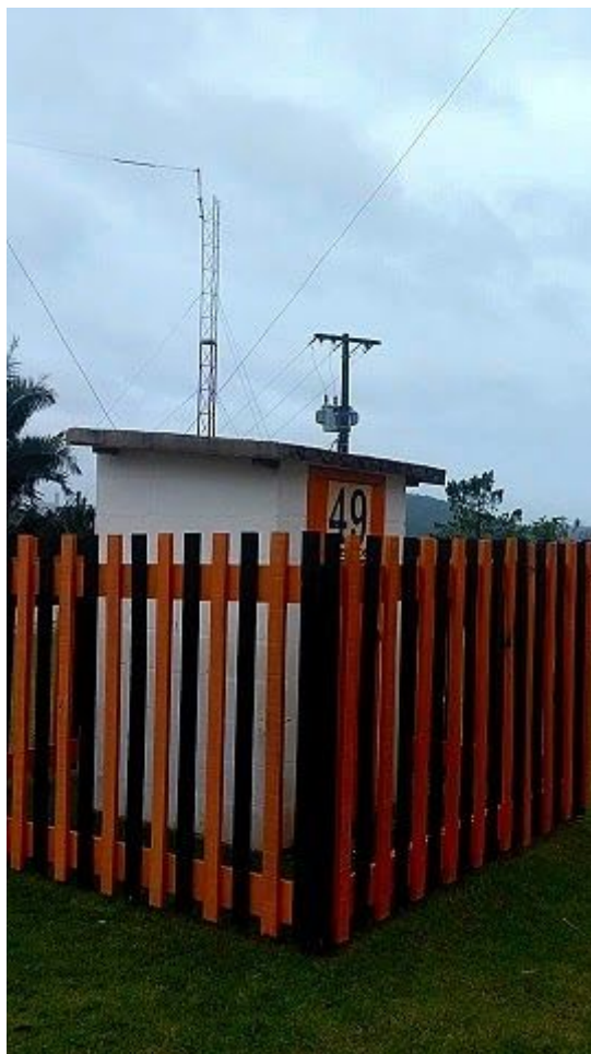
Photo: Box where the coupler for the 49M antenna is housed.
