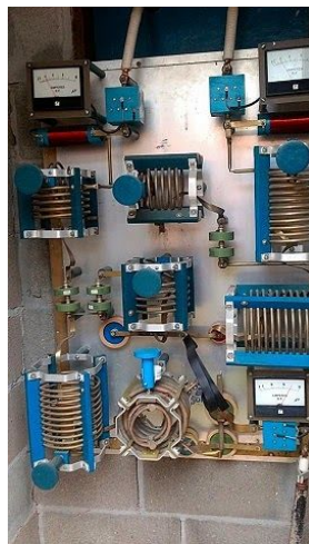
Photo: Coupling system of one of the antennas.
